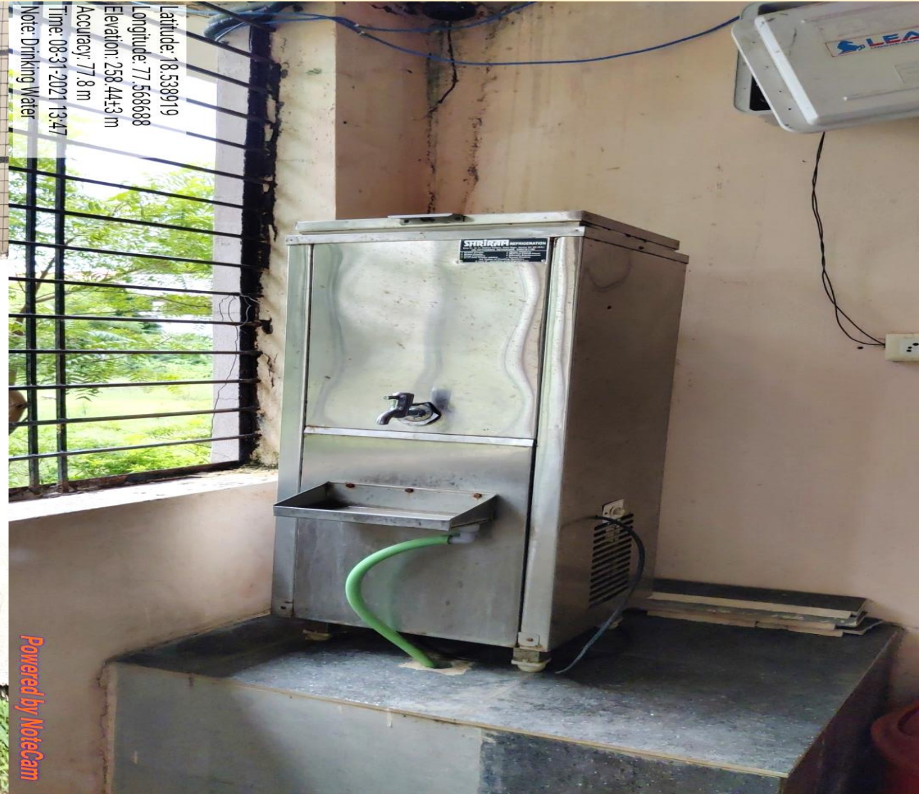
R O Drinking Water Facility
