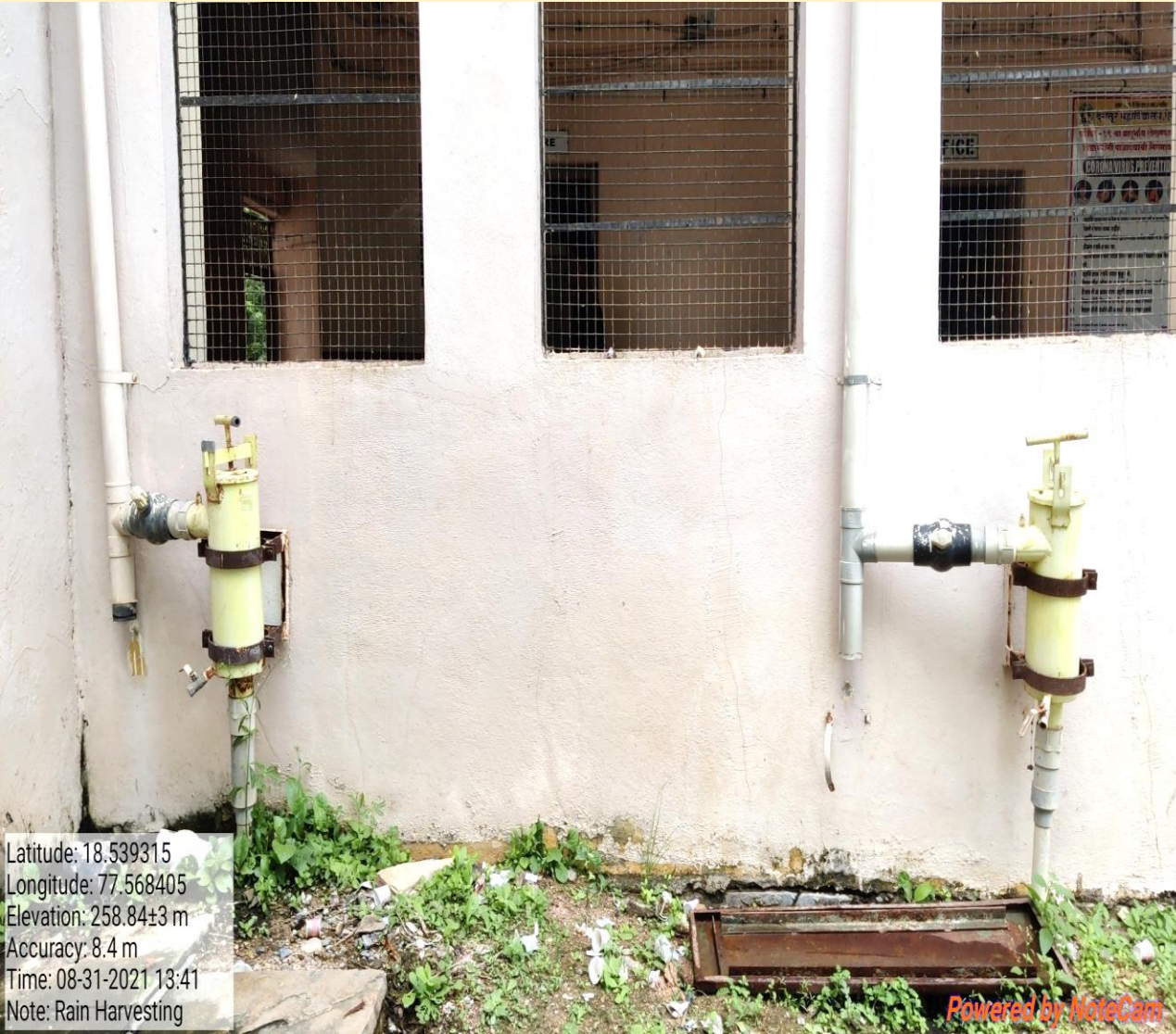
Rain Water Harvesting
